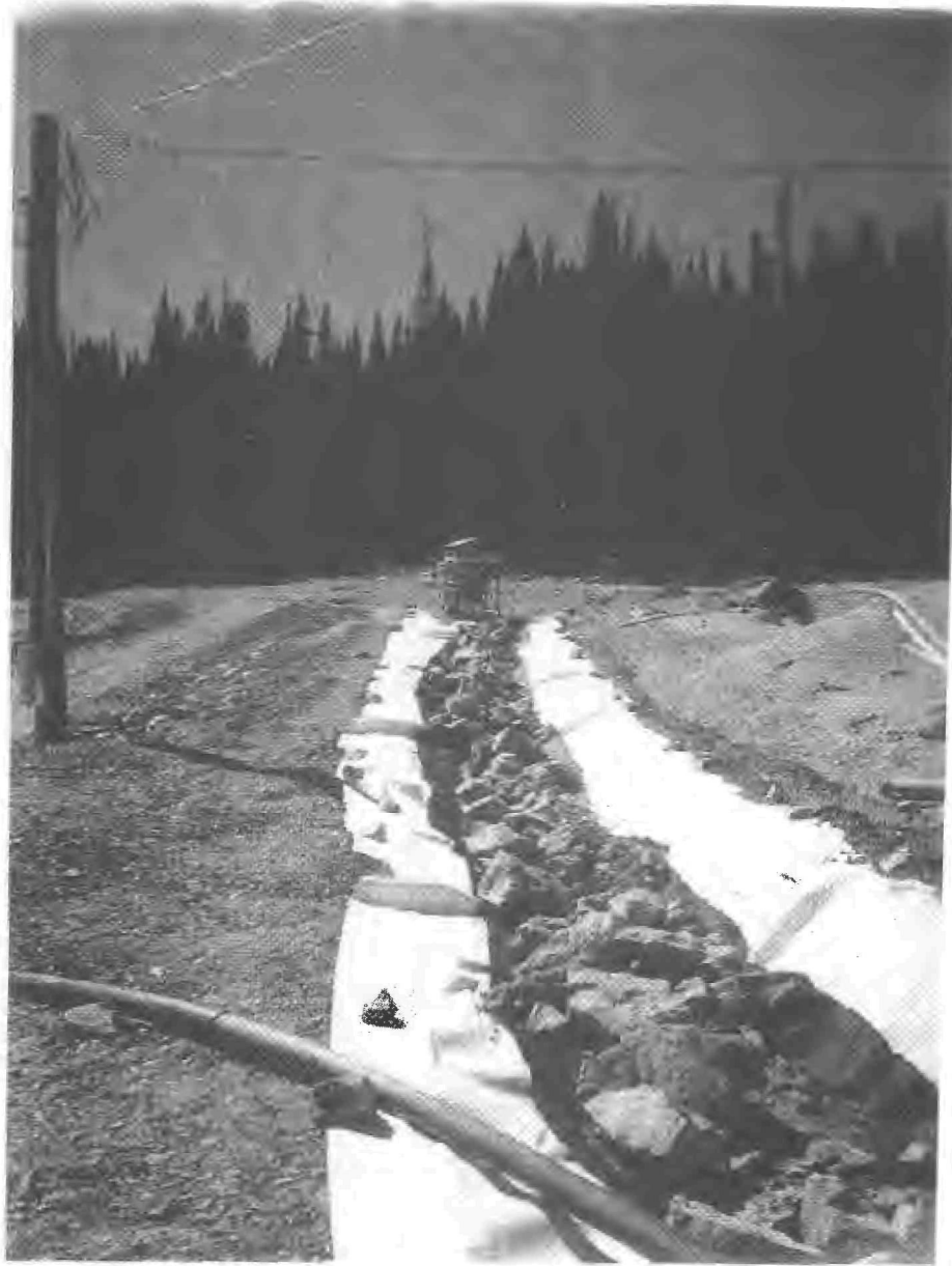
Photograph shows rock trench and plastic liner in foreground and Aquafix system in background.
